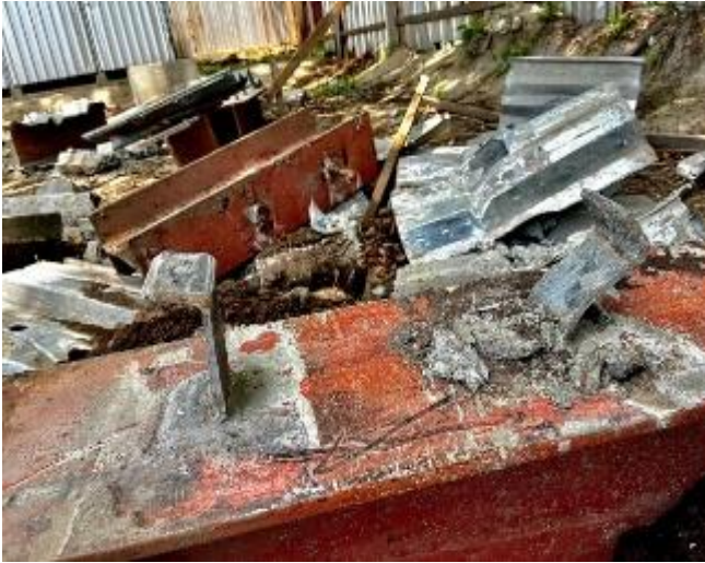
Fig. 8. Post-test condition of U-shaped channel connector
