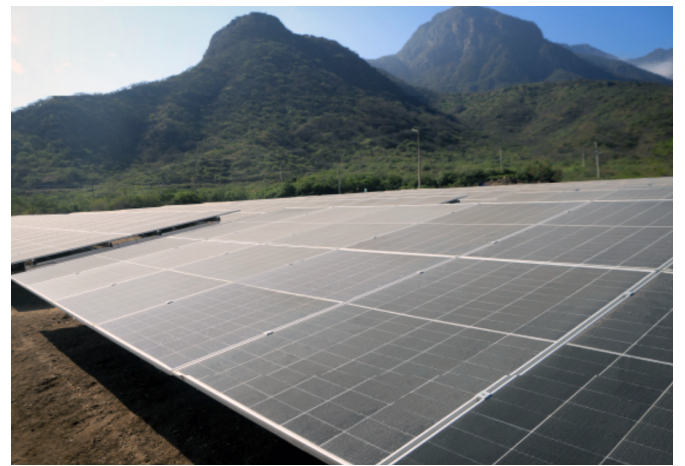
Fig. 2. Solar Panels of the Carhuaquero Photovoltaic Solar Plant
