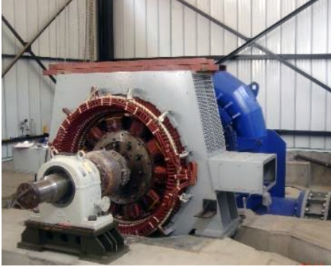
Fig. 4. The Turbine and the Electric Generator
