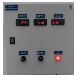
Fig. 2 Distillation Column Control Panel
