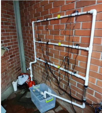
Figure 3. Assembly of the functional prototype with its automated electrical network
