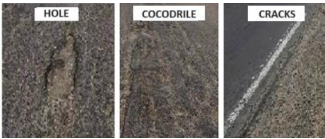
Fig. 6. Failures found in the pavement with different severity.
