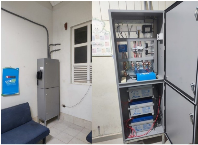
Fig. 3. Client station cabinets completed in initial phase (Hospital and Health network of Condorcanqui): a) Telephone for VoIP communication installed. b) Internal wiring for battery power consumption, connection to Access Point, ATA and batteries.
