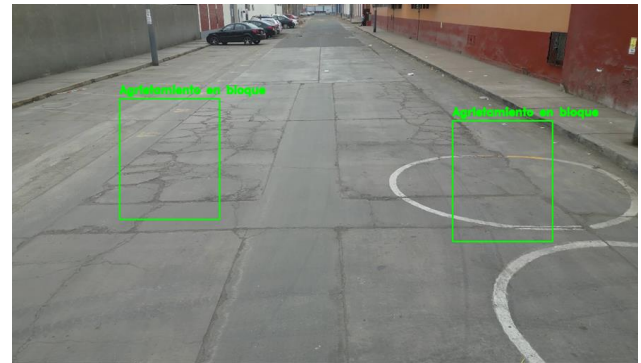
Fig.11. Block Cracking Failures Detection via Drone Camera
