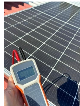
Figure 4: North-facing solar panel
