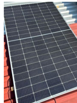
Figure 5: South-facing solar panel
