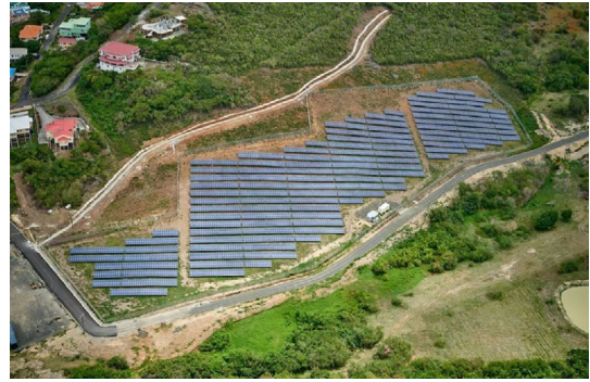
Figure 1: Vieux Fort Solar Array Installation [12]
