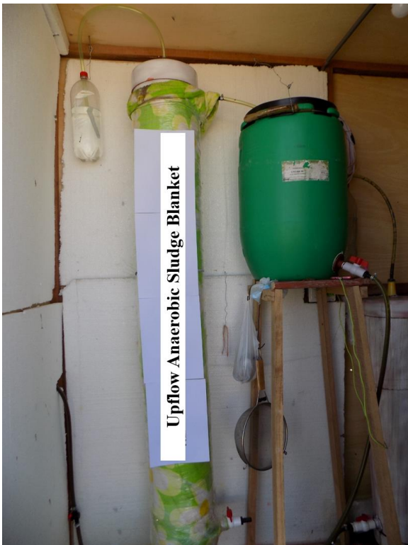
Fig. 3 Upflow Anaerobic Sludge Blanket of rigid plastic polyvinyl chloride installed in the facilities of the Mario Eyzaguirre Yáñez municipal slaughterhouse in Tacna.
