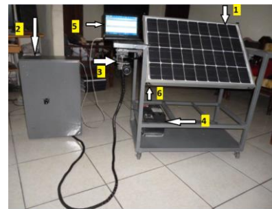
Fig. 5 PV System Components. [8].
