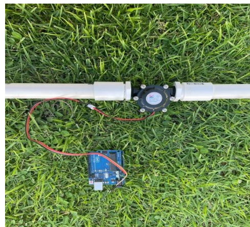
Figure 14. Closeup of turbine connected in a piping system
