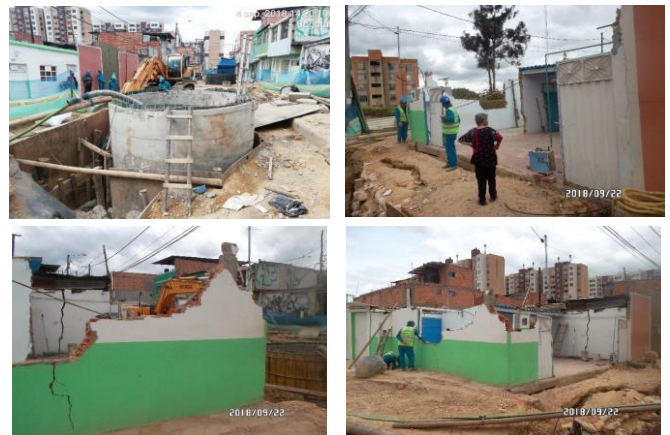
Fig. 1. Surface deterioration of the physical environment caused by the excavation of a tunnel with trenchless technology for the construction of an 80-inch diameter sewer in the southwest of Bogota, D.C., Colombia. Courtesy of Dicefin S.A.S. (2019)
