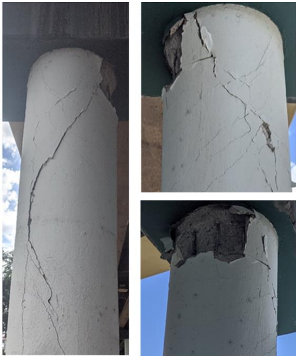
Fig. 4 Earthquake Damages to Viaduct Bridge Column in Mayagüez, Puerto Rico (source: Vidot, A. & Montejo, L.)
