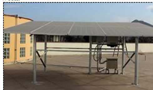
Fig. 3. A 3.25-kWp Solar PV System (Sunny Portal Web)
