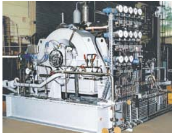
Figure 2: Turbine-generator Siemens SST-200
